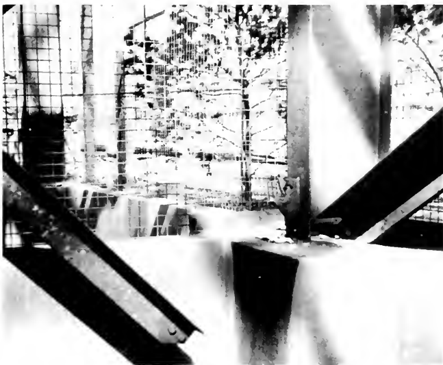
Photo 19. Sylmar Converter Station, radio interference structure. Broken diagonal bracing connection.
